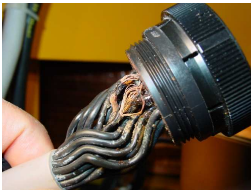
Burn connections of the center coils
